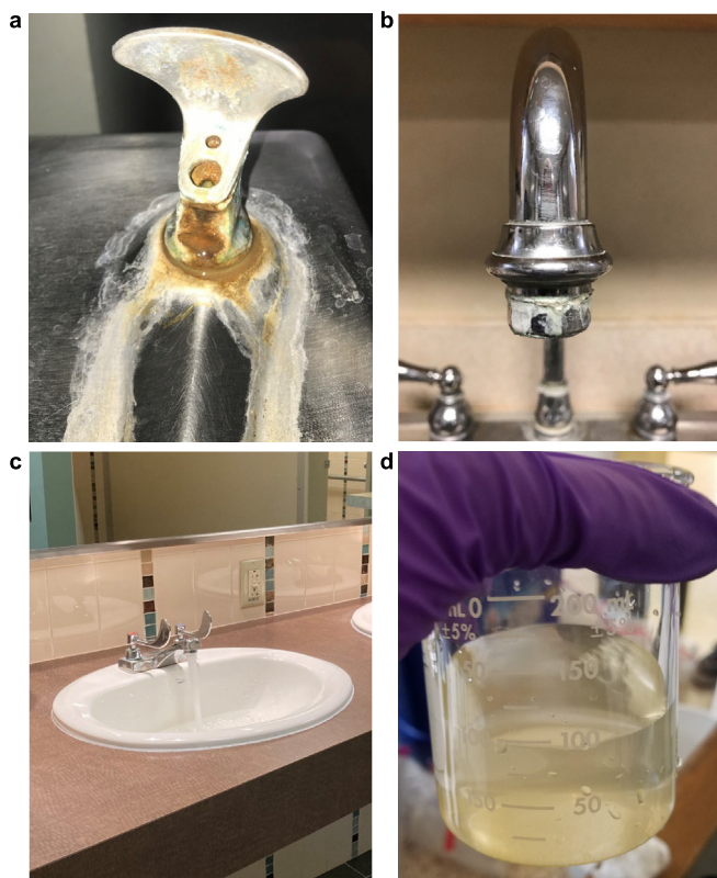
Fig. 2. Various fixture conditions: a drinking water fountain bubbler in building A (a), a breakroom faucet in building C (b), a 2nd-floor bathroom faucet was flushed for 7.7 h in building D (c), and colored water from building D in March 2020 (d). After the buildings were reopened, the drinking water fountain from building A was replaced with a new drinking water fountain containing filters.
